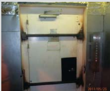
Elevator door bolted
